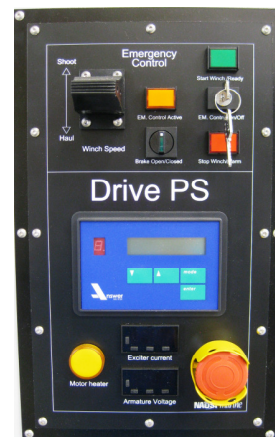
Control on Cabinet
