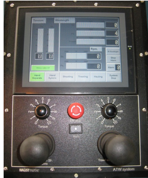
Winch cabin control
